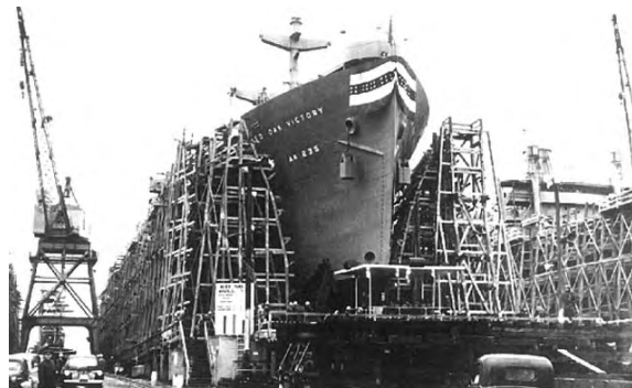
The SS Red Oak Victory Ship being constructed, Richmond Museum of History Collection.
