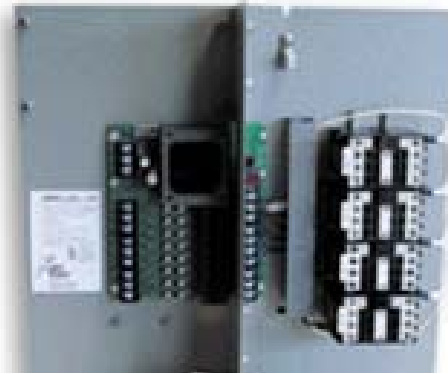
Figure A-13: Interior of a Lighting Control Panel (Source: Watt Stopper)
