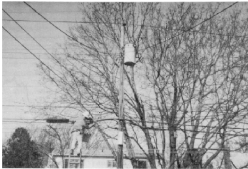
FIGURE 16. Two different splicers working in residential section illustrating (a) no transformer and (b) presence of transformer.
