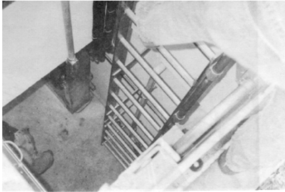
FIGURE 17. Entrance to typical NYNEX underground controlled environmental vault (CEV)
