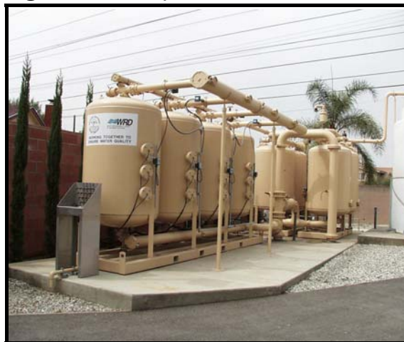
Figure 4: Century Well Pilot Test Vessels
