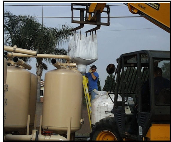
Figure 2: Loading Arsenic Treatment Media
