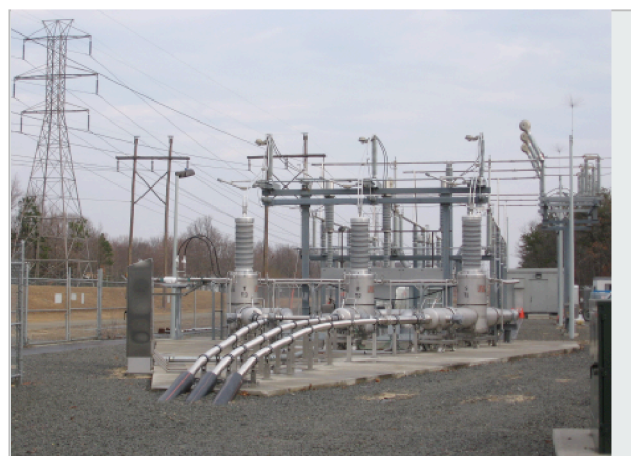
▲ The world's first HTS power transmission cable system. The three cables shown entering the ground can carry as much power as all of the overhead lines on the far left.
