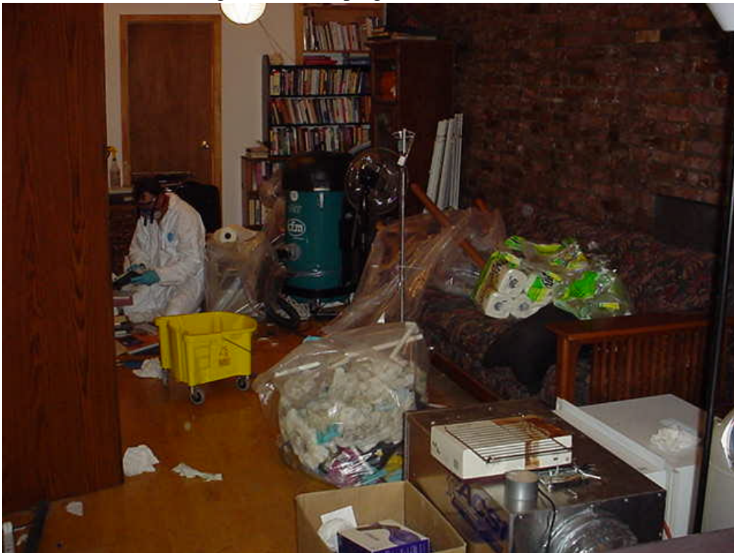
Vacuuming and Wet Wiping Dust from Personal Items
