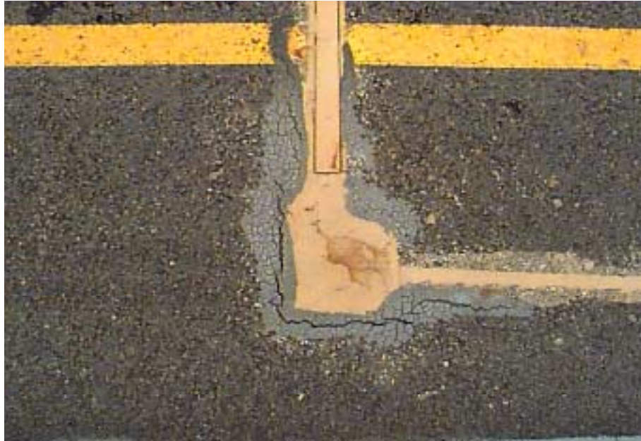
Figure 6A, Cracking Along End of Sensor Where Cables Exit Through Conduits
