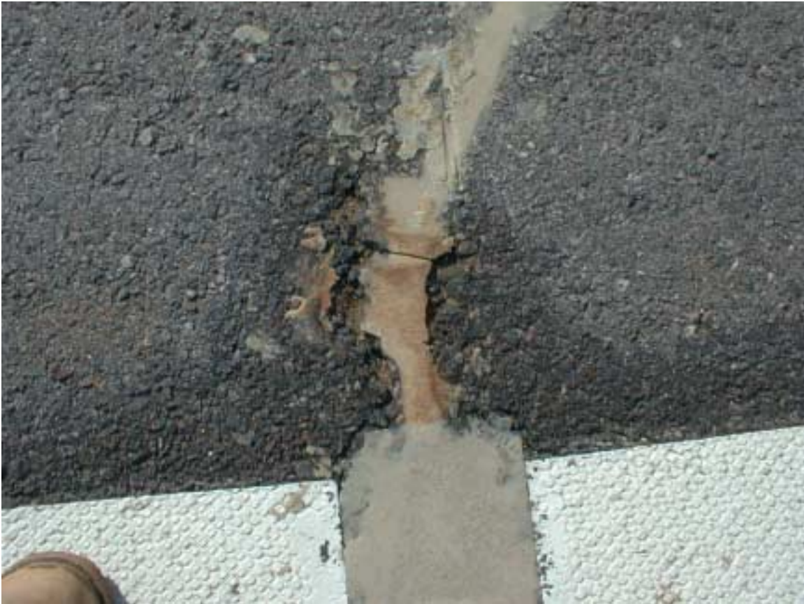
Figure 6B, Cracking and Pavement Deterioration at End of Sensor in Lane 2
