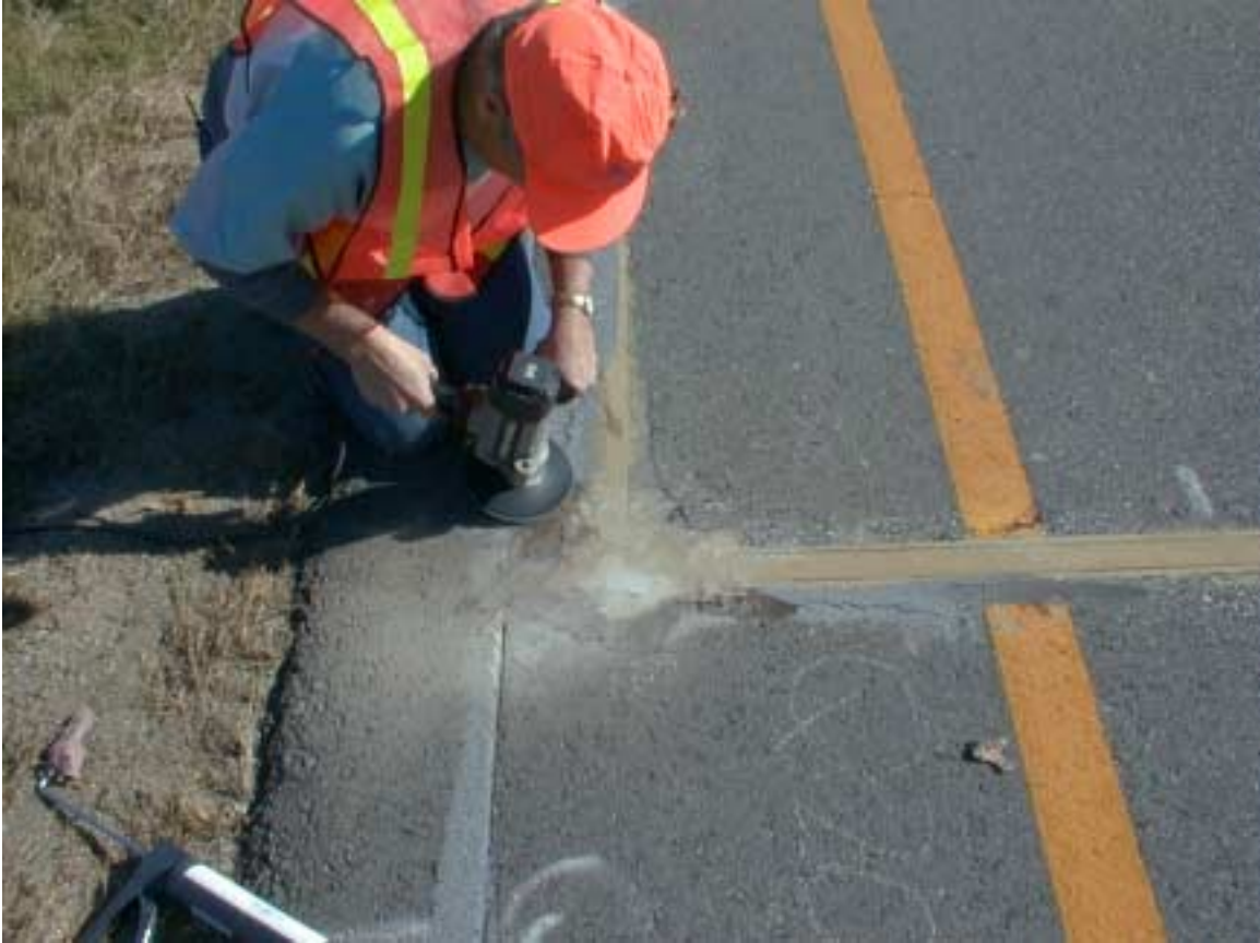
Figure 7, Grinding the Edge of Grout that Has Risen Above Shoulder Pavement Surface
