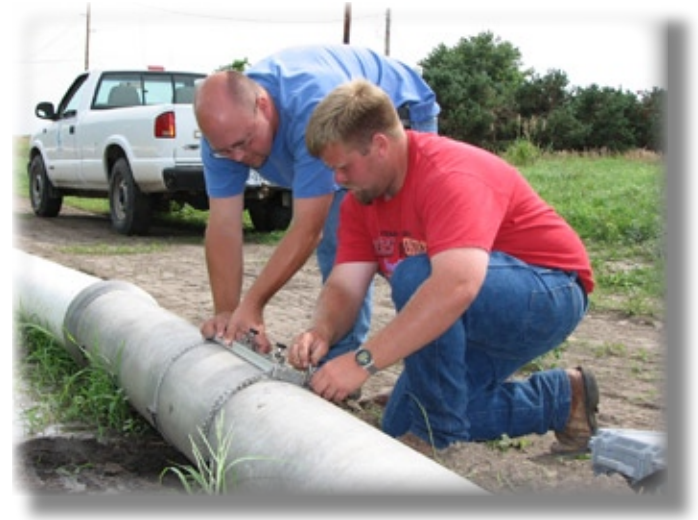
Photo courtesy of Kearney Hub NRCS Water Quality Specialist Curtis Scheele (left) trains Earth Team Volunteer Josh Hohanson how to install and operate an ultrasonic flow meter on an irrigation pipe. Scheele submitted the winning Chief's Field Award nomination highlighting the interns' help.
