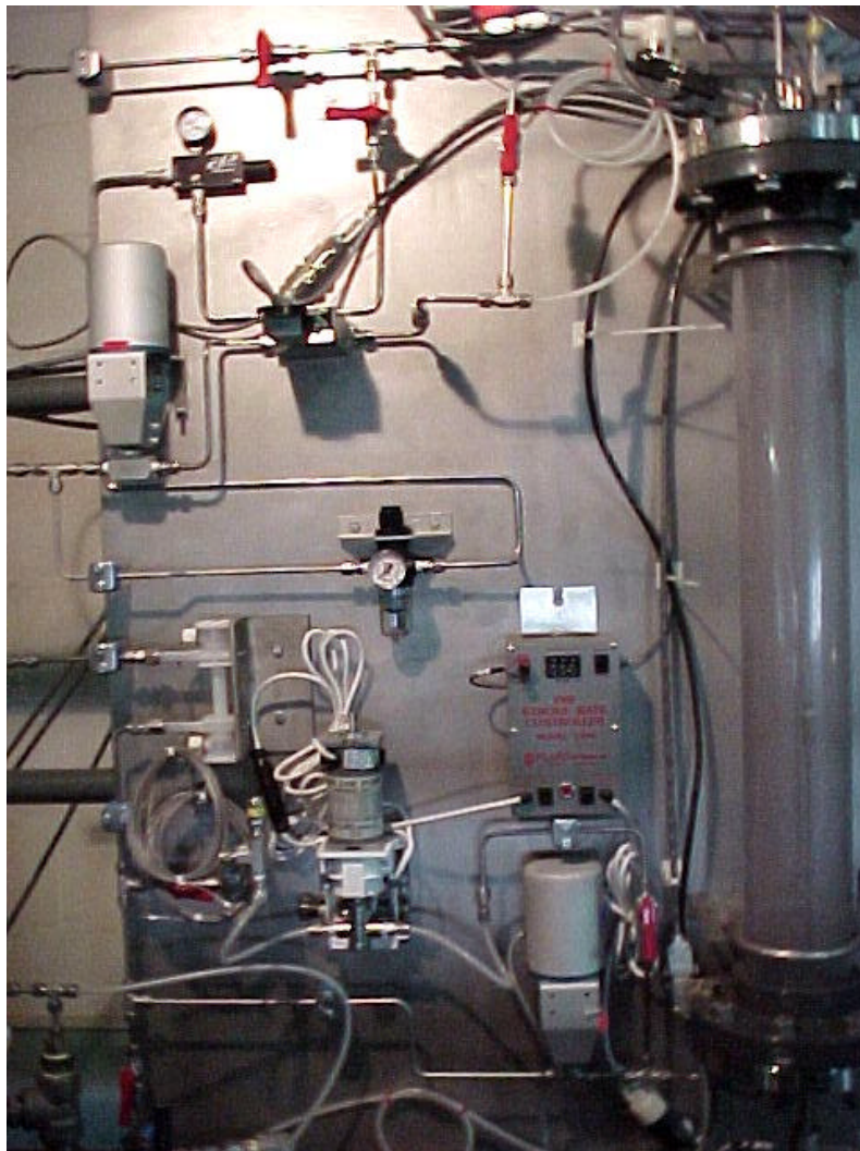
Fig. 3.7. Gas disengaging equipment.
