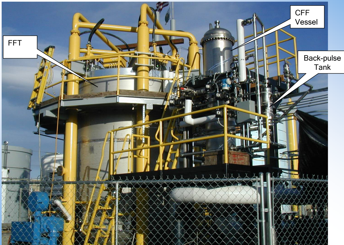
SWPF Cross Flow Filter Full Scale Test
