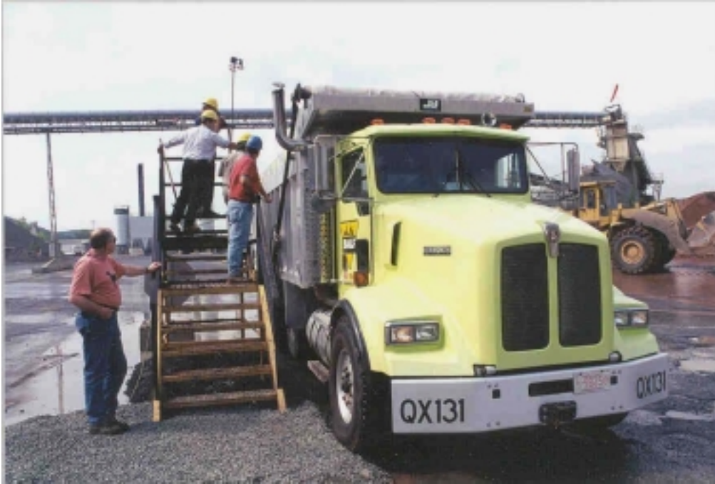
Photo #9. Department Personnel Use Infrared Camera to Look at Truckload of HMA.
