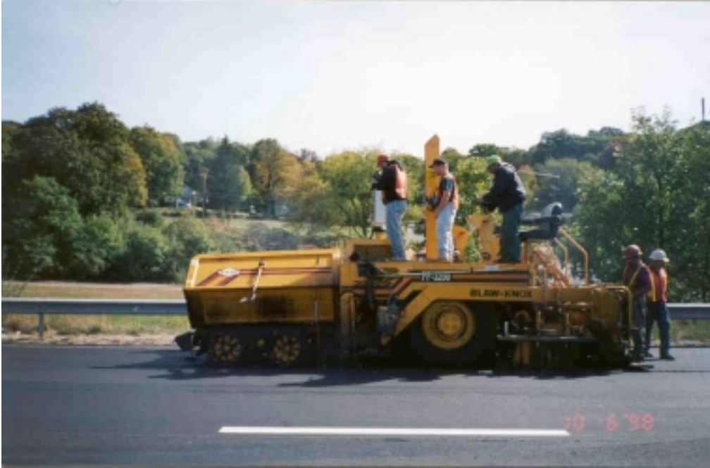
Photo #5. Infrared Video Being Recorded From Top of Blaw-Knox PF-3200 Paver at Site 3.
