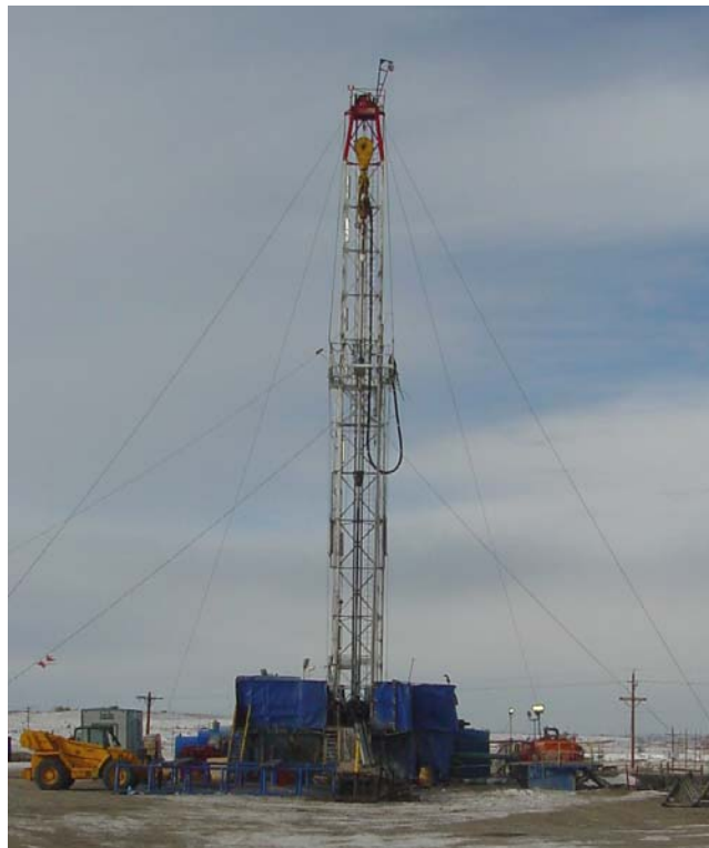
Figure 44. RMOTC Rig #1, Teapot Dome near Casper, Wyoming
