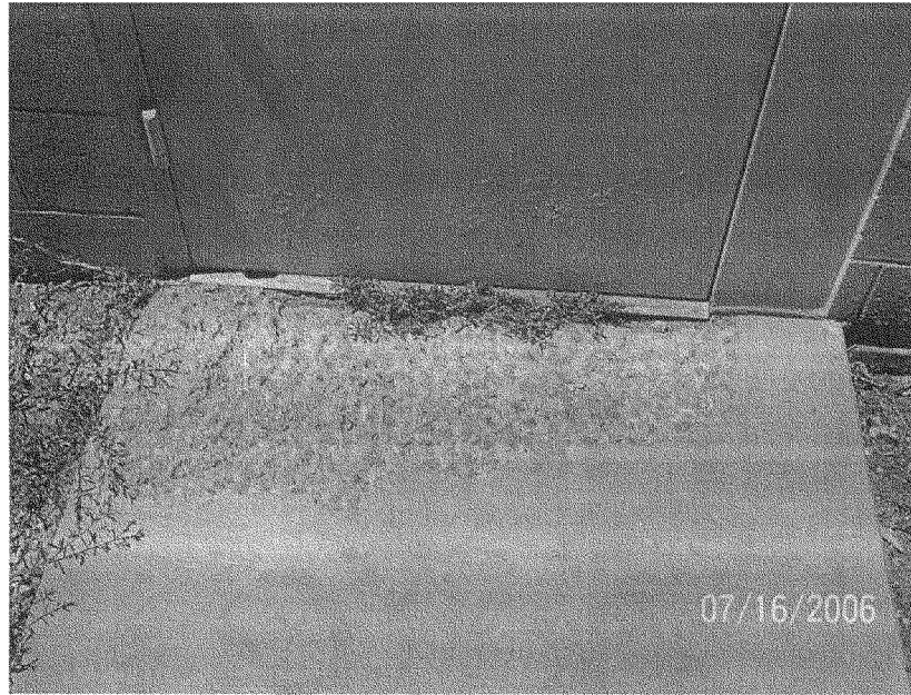
Concrete has to be scraped out to permit opening of the door – which is sinking at a faster rate than the concrete slab outside
