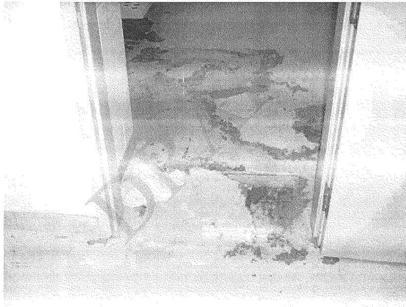
Stains from sewage in the cell, spilled over from the toilet connection at the sink-toilet combination unit
