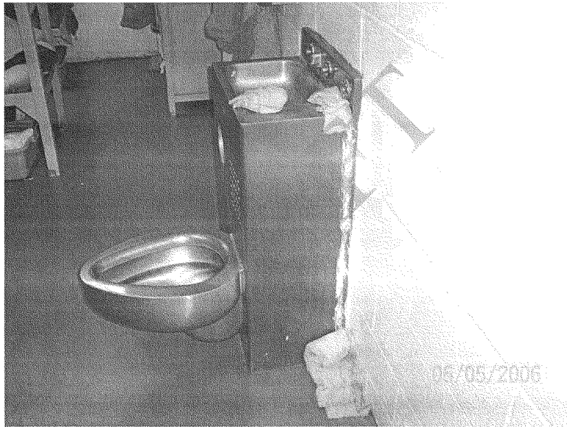
Wadded up towels on the floor to cleanup the sewage spillover
