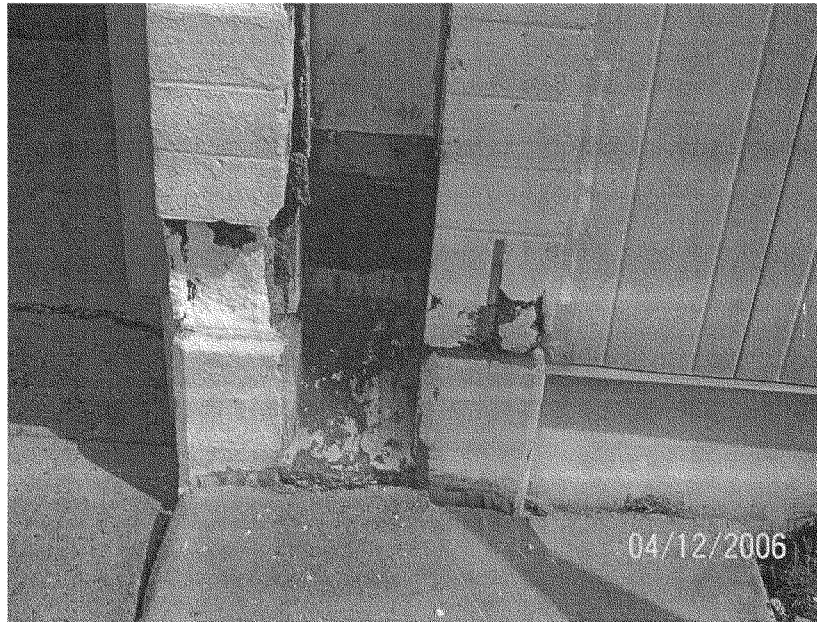
Weathered and crumbled concrete fins
