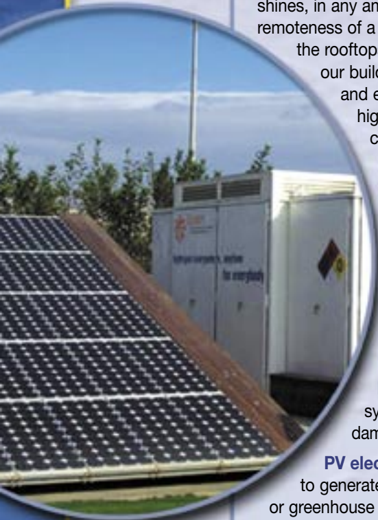
A PV system at SunLine Transit Agency in Thousand Palms, California, provides electricity to the Stuart Energy electrolysis unit on the right for producing hydrogen from water. (Richard Parish, PIX10719)
