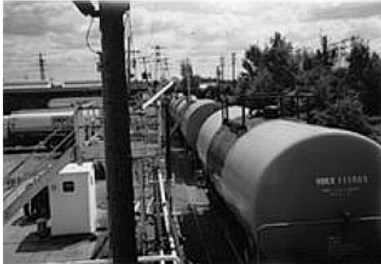
Figure 22: Rail Tank Car Loading Facility (24).
