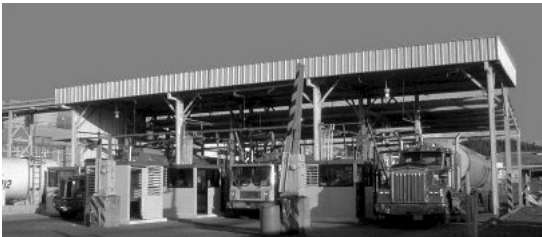
Figure 21: Tank Truck Loading Rack (24).
