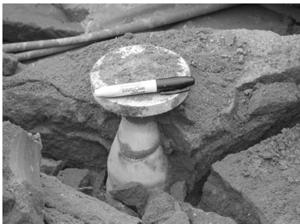
Figure 4-27. Simulated debris in Pool 1 filled and covered with Stabilization grout. (Marker for reference.)
