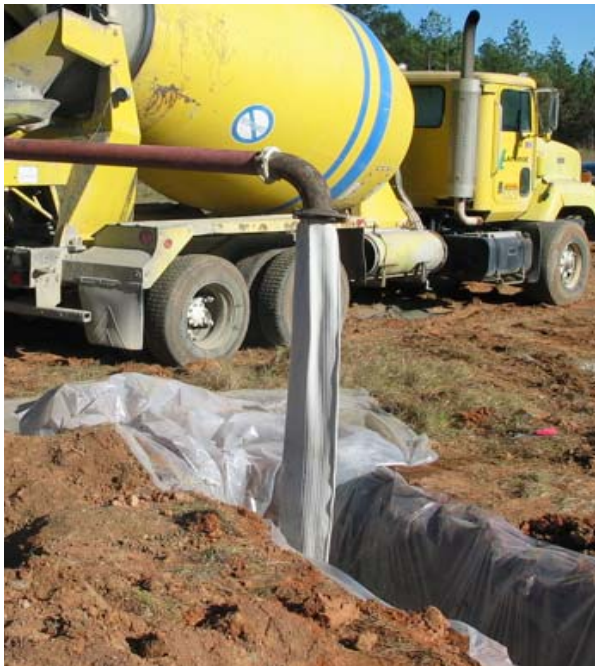
Figure 4-11. Capping grout, SRG9, discharged into Trench 3 from a two-foot drop through a tremie.
