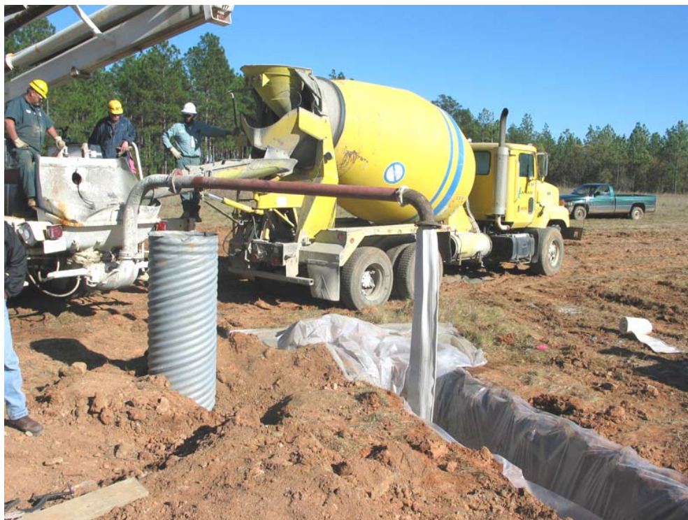
Figure 3-22. Placement through a 5 inch metal line with a flexible tremie at the discharge.
