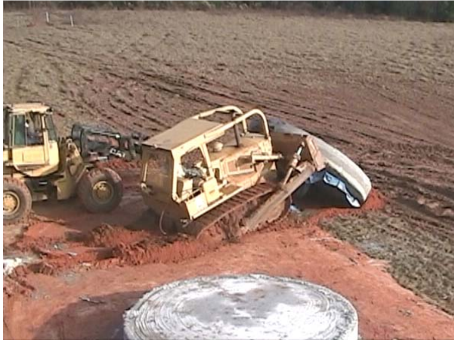
Figure 3-31. Demolition of the pool 1 monolith 5 days after the final Capping Grout pour.
