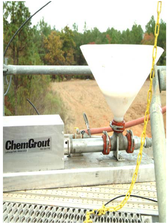
Figure 3-28. Equipment/riser grout funnel hopper which contained a screen to remove lumps prior to pumping.
