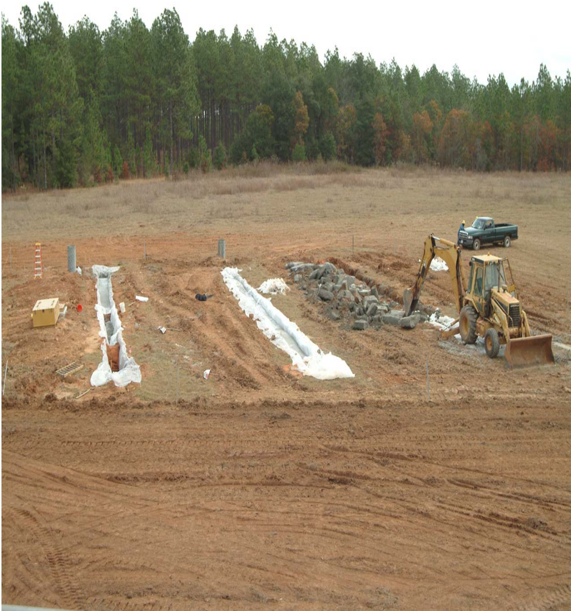
Figure 3-1. Burma Road Landfill test location for the Hanford grout scale-up tests. The three 80-foot long trench forms are shown. The first trench to be completed is being dismantled.
