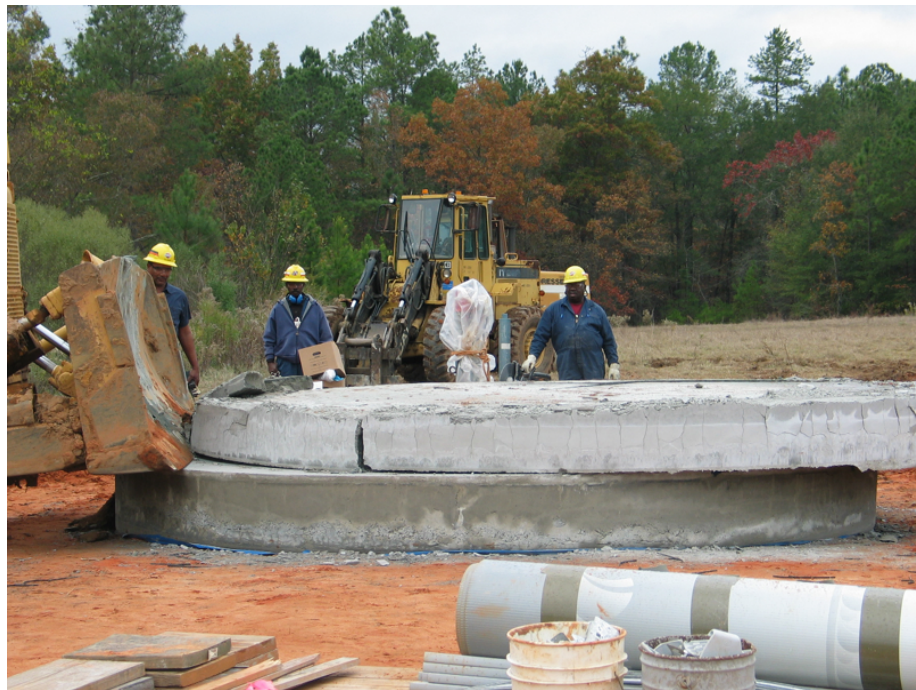
Figure 3-32. Demolition of the pool 2 monolith 5 days after the final Capping Grout pour.
