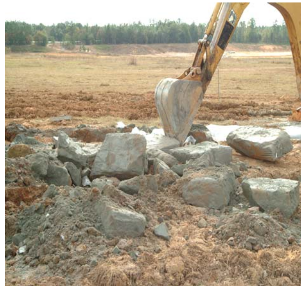
Figure 3-30. Size reduction of the grouts poured in the trench forms after curing for 5 to 10 days.
