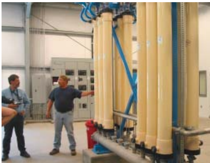
Hoopa Valley Tribe - microfiltration treatment
