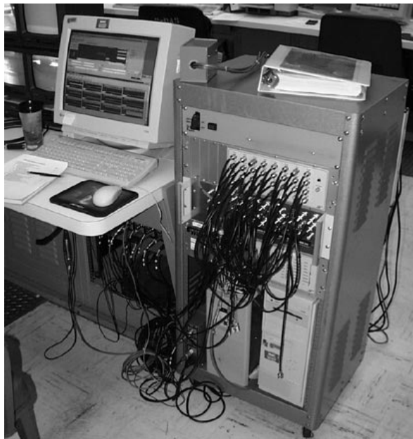
Figure 12. PSC computer used during HXFE/VFS testing.
