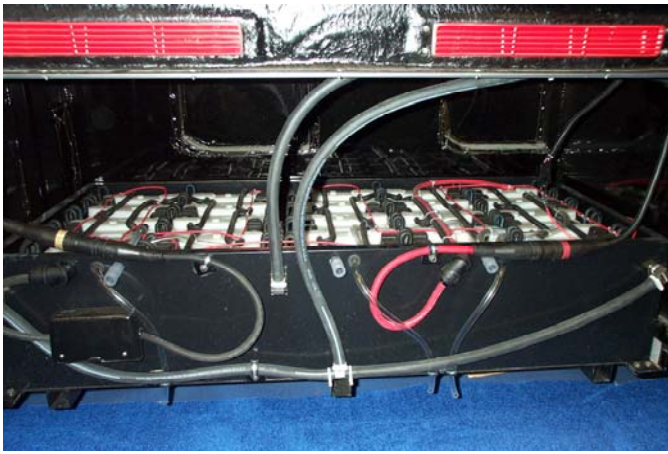
Water cooled thermal management system on a battery electric bus.
