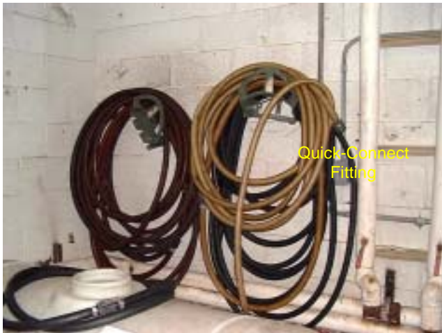
Photo No.2 – Delivery Hoses
