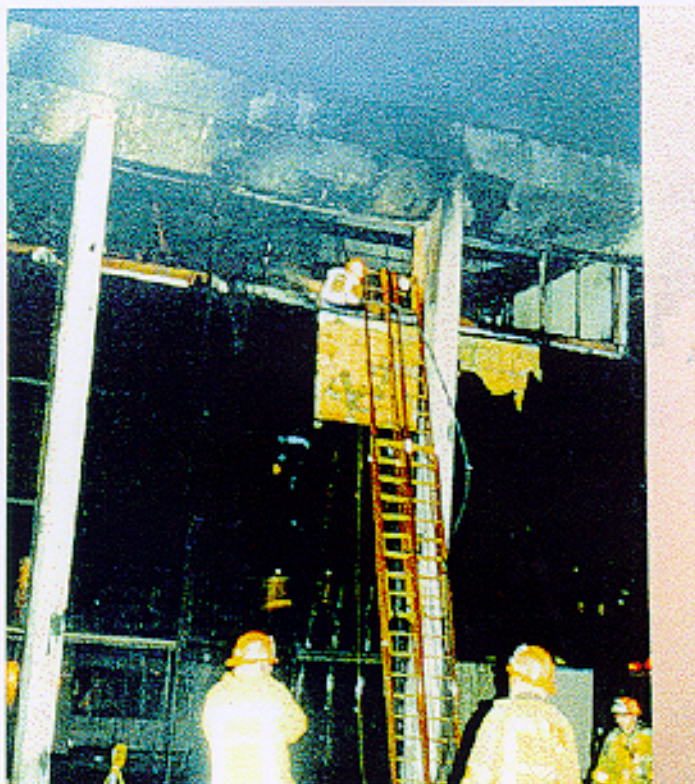
3-14: Structure fire, California State University, Northridge, Science Building
