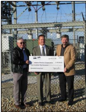
Adams Electric Cooperative Board President Rick King and General Manager Jim Thompson accept a check from Illinois Rural Development Director Doug Wilson for a grant to help purchase a wind turbine. The check was presented at the substation where electricity will be uploaded from the wind turbine just down the road.
