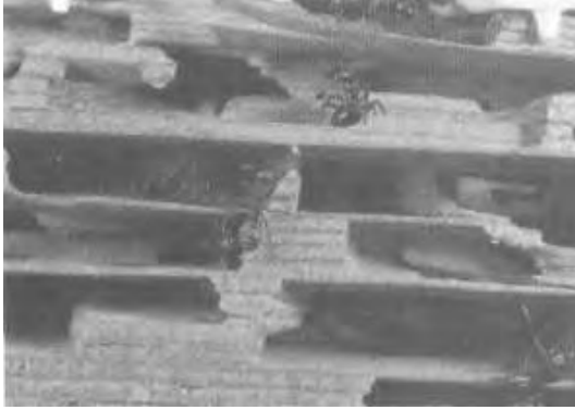
Carpenter Ant Galleries
