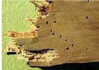
Powderpost Beetle Damage
