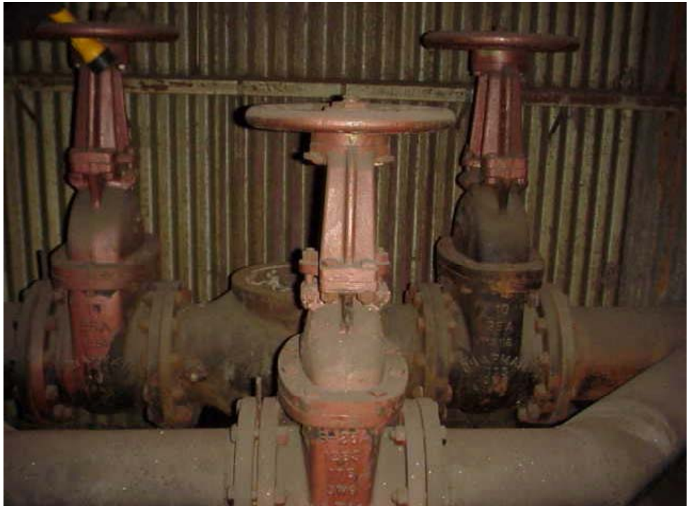
Picture 6 – Coke Oven Gas Line Balance Piston Valve
