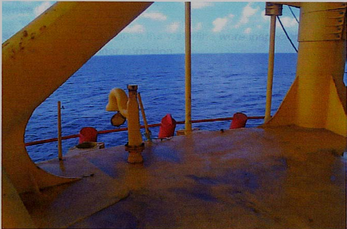
Picture 2.6-2 – Missing or Bent Handrails due to Hurricane Lili
