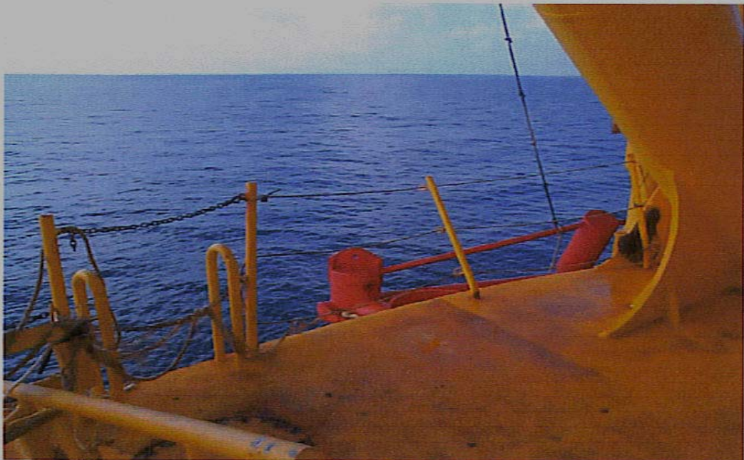
Picture 2.6-3 – Missing or Bent Handrails due to Hurricane Lili
