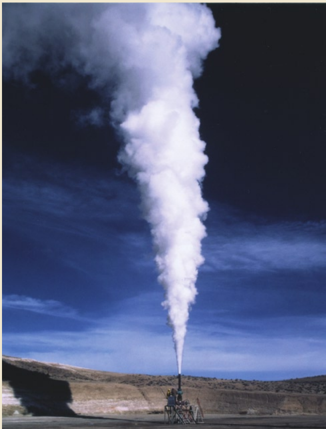
First geothermal well drilled at Coso geothermal area, south-central California, by private industry. It, together with a few other wells, has been developed to feed steam into the initial powerplant.
