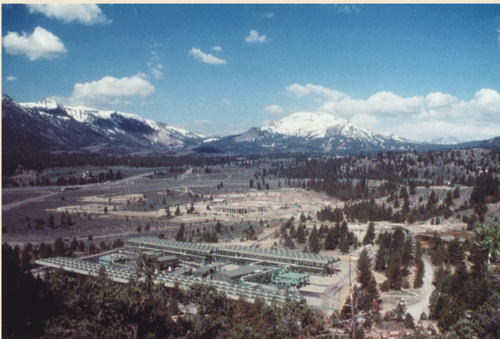
Binary-cycle geothermal powerplants near Mammoth Lakes, California. Mammoth Mountain in background on right. (Photograph by Edward Evans.)
