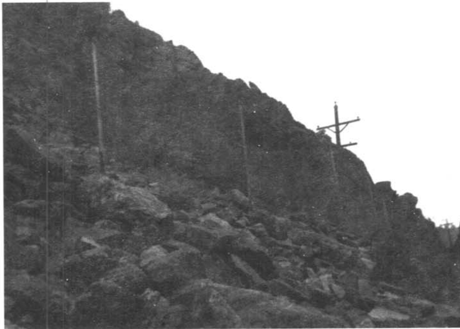
Figure 5.—Colorado flex post fence.
