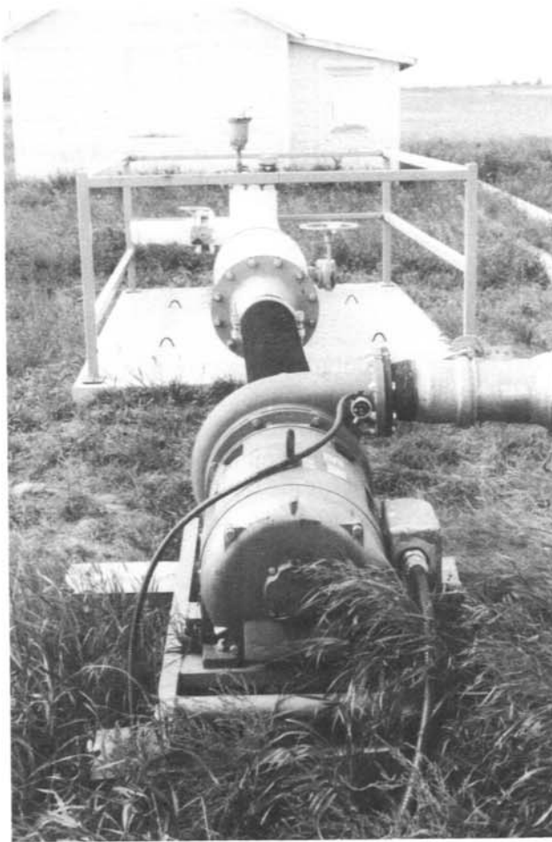
Figure 2.—Electric pump site.
