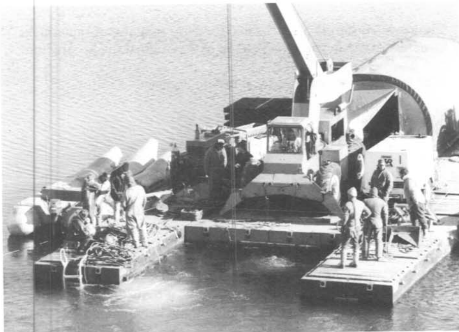
Figure 3.—Hyrum Project, Utah. Installation of new intake structure extension in progress. The crane shown in the photograph is lowering the intake structure as it is guided and secured in place by divers.
