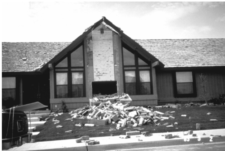
Figure 7-1 Chimney damage. Photo Courtesy National Information Service for Earthquake Engineering, University of California, Berkeley
