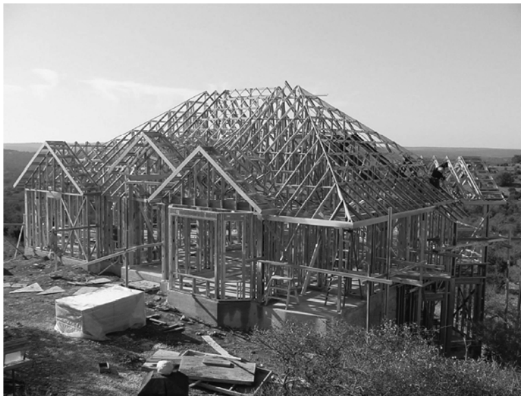
Figure 5-13 Cold-formed steel house under construction. Photo Courtesy of Dietrich Metal Framing -- a Worthington Industries Company
