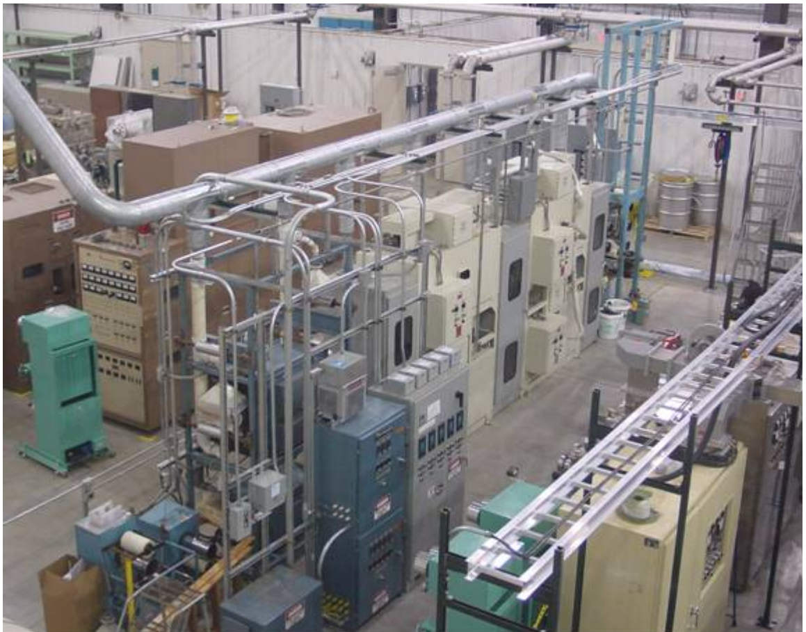
Figure 2. Conventional pilot-line installation at ORNL.
