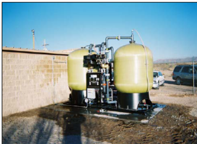
Figure 4. Arsenic adsorption treatment plant at Desert Sands, NM.
