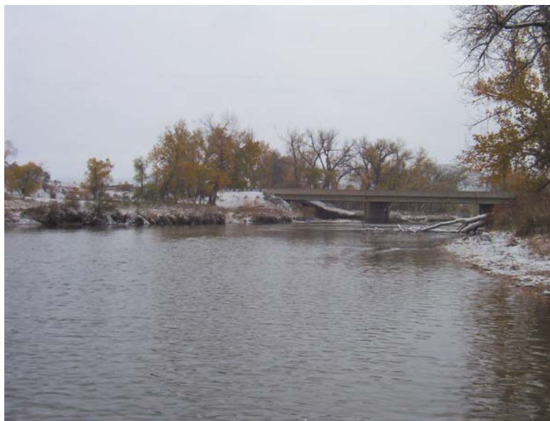
Figure C3. Tongue River at Birney Day School Bridge site from left bank near cross section 1. View is looking upstream at cross section 2 and Birney Day School Bridge. Photograph taken October 22, 2002.
