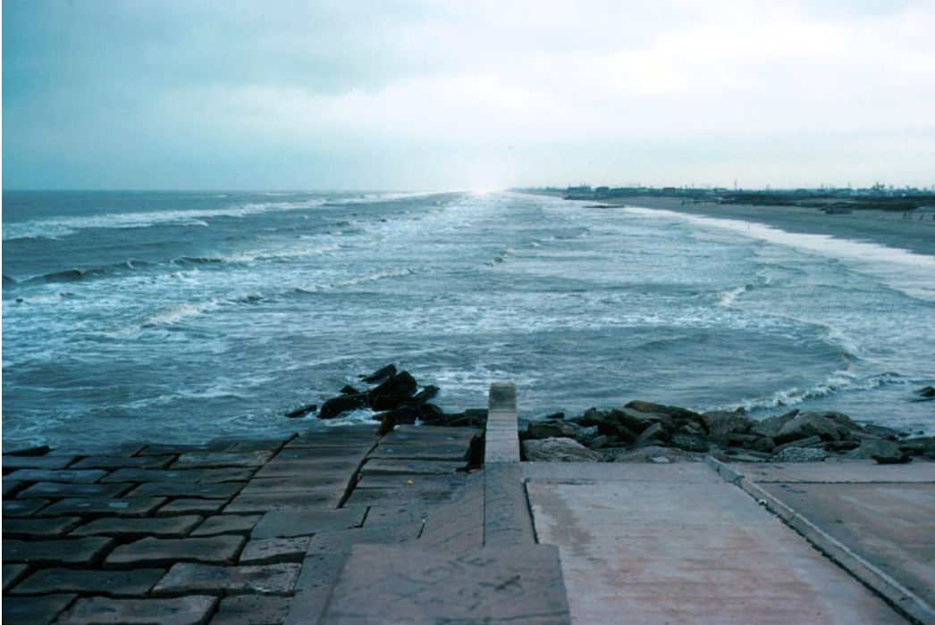
Figure 25. West end of the seawall at Galveston, Texas. The concrete ramp (right foreground) was the road leading to the beach in the mid 1960s. Since then the beach has eroded more than 150 m.
