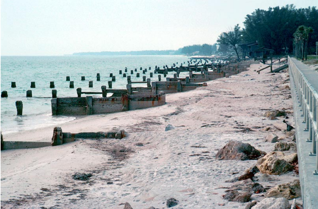
Figure 21. Multiple structures including a seawall, riprap, and failed groin field have been unable to stop erosion at Longboat Key, Florida. Later these structures were removed and the beach was nourished.
