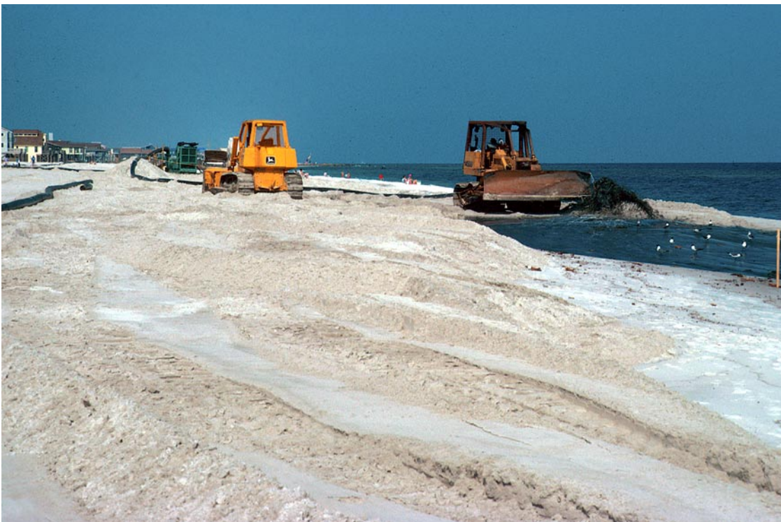
Figure 18. A beach nourishment project near Gulf Shores, Alabama. Accelerated erosion in front of the beach houses was attributed to construction of an artificial channel and jetties.
