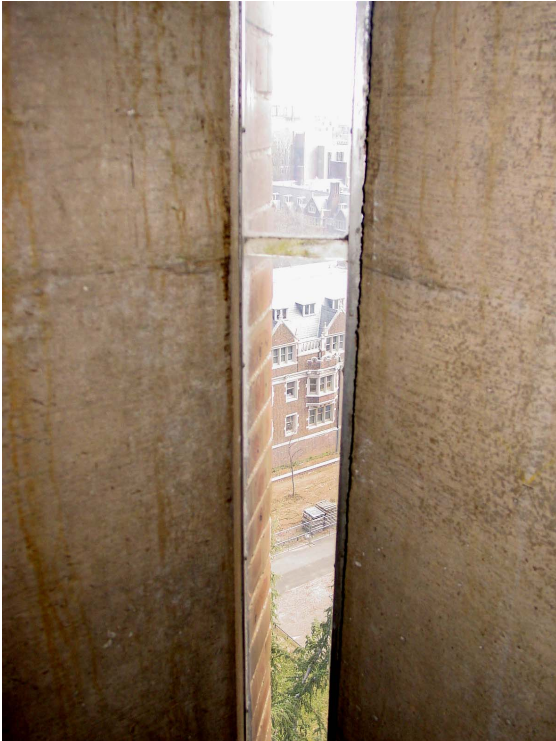
Goddard Building, detail of strip window in western stair tower, looking northwest Emily T. Cooperman, photographer, 2008
