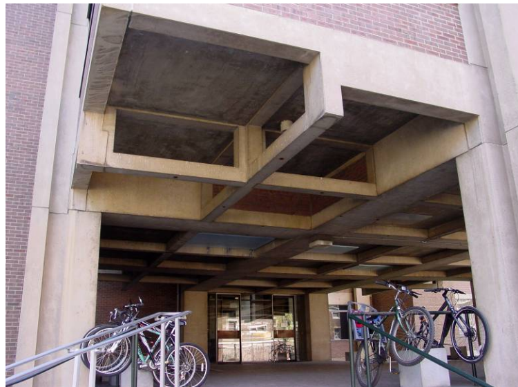
Richards Building, entry, looking southeast (top), and entrance detail showing the Vierendeel truss system (bottom) Emily T. Cooperman, photographer, 2008
