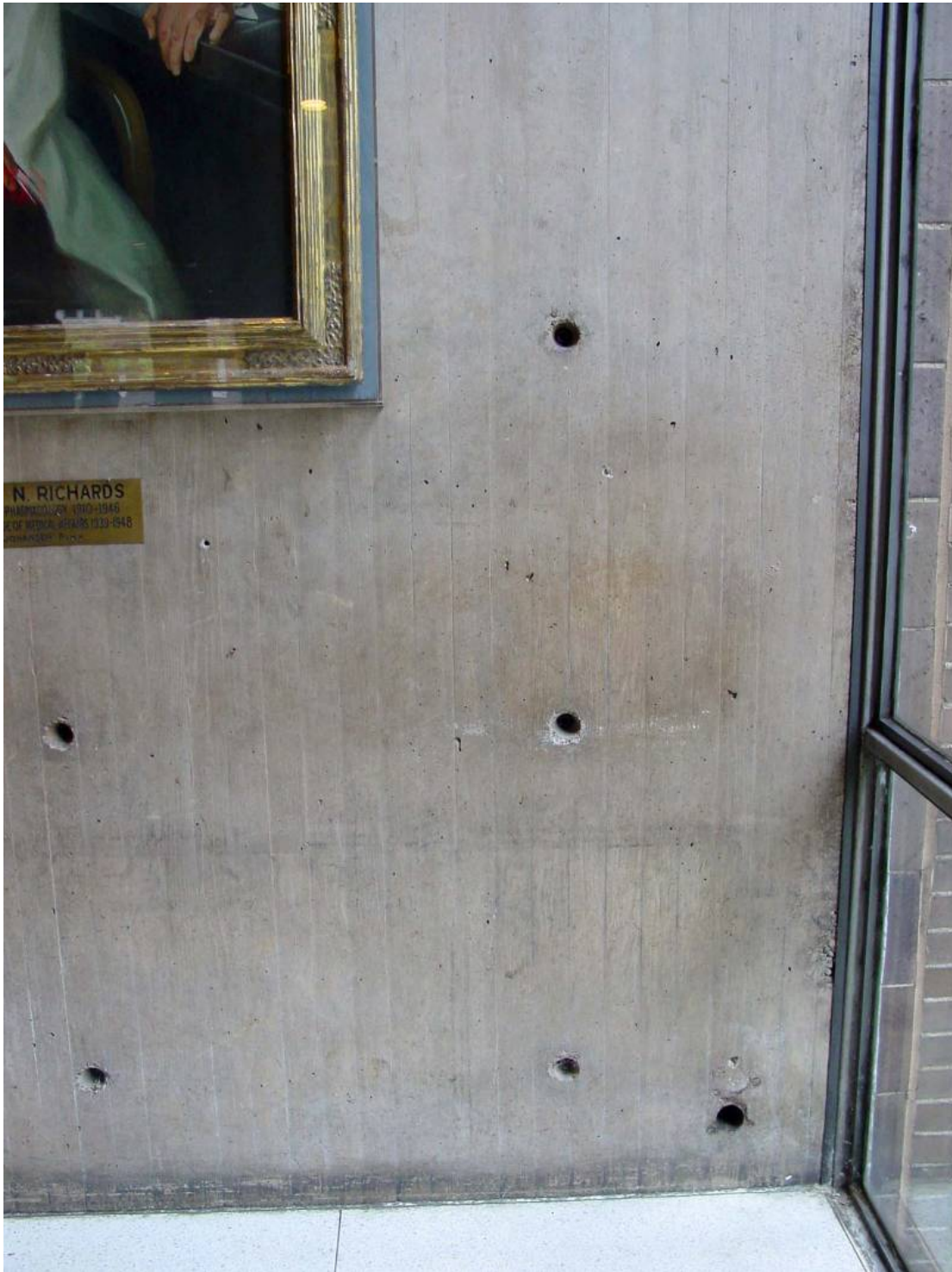
Richards Building, lobby detail, poured-in-place, reinforced concrete treatment, looking south Emily T. Cooperman, photographer, 2008
