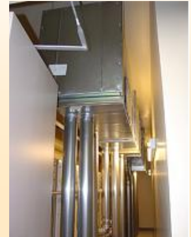
Heat Recovery from Dryer Vents
