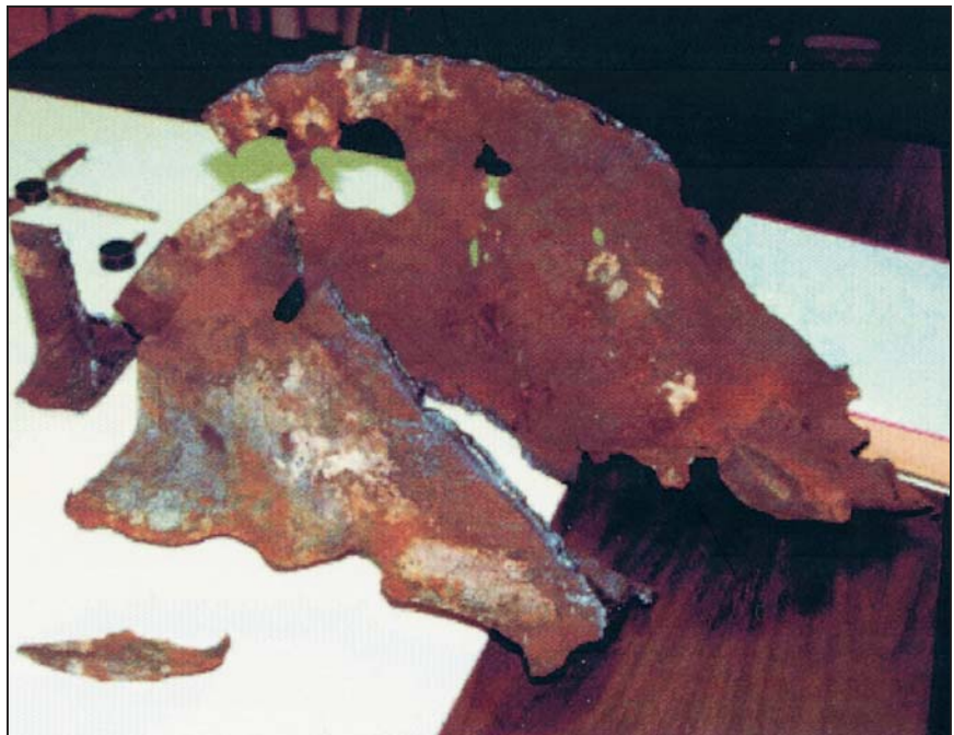
Figure C-1 Eroded A36 wide-flange beam.
