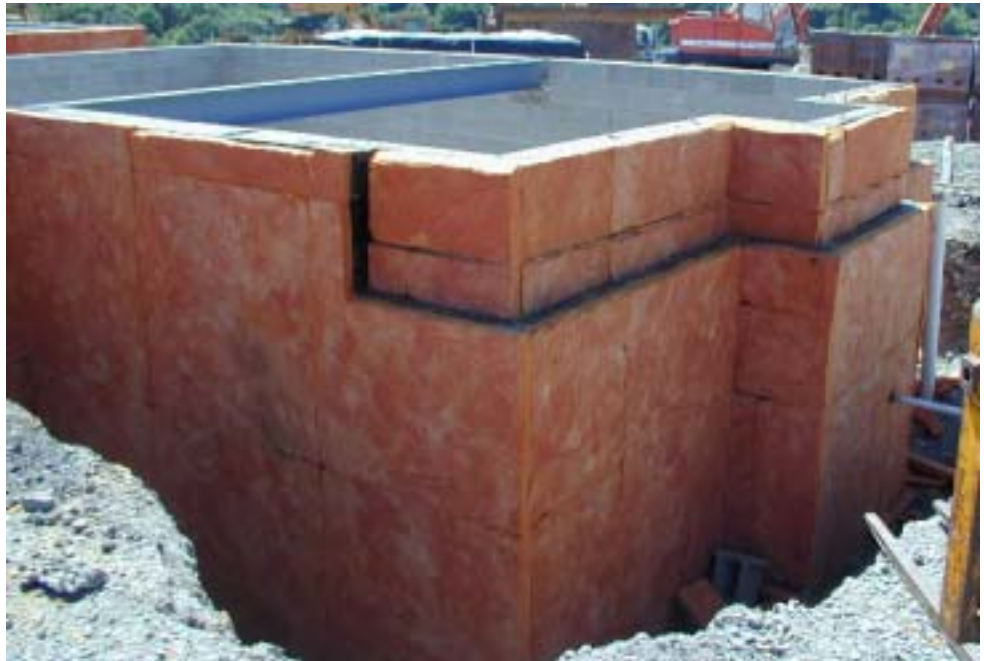
Figure 1. The semi-rigid fiberglass board insulation, 2 and 3/8 inches thick, provides R-10 thermal performance and water drainage at the exterior of the foundation wall. It was applied over a dampproof coating to the height of the sill plate. The exterior edge of the brick or wall sheathing above the board was designed and installed so that the edge would lay flush with the foundation wall, thereby protecting the top edge of the insulation board.
