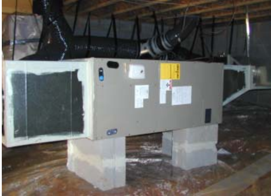
Figure 7. Locating mechanical equipment responsible for air movement in a conditioned space, such as this conditioned crawlspace, means that it is not subject to the cold and extreme hot and humid circumstances that it would experience if it was located in an attic, vented crawlspace, or the outdoors.
