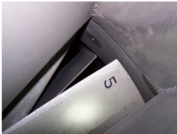
Figure 8. Probe installation on the axial vane fan.
