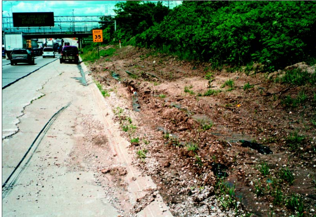
Figure 3. Example of dirt and gravel from utility construction on highway shoulder.
