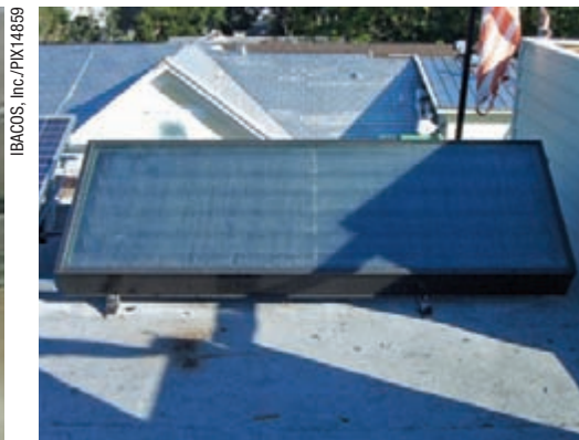
A solar thermal hot water system preheats incoming water.
