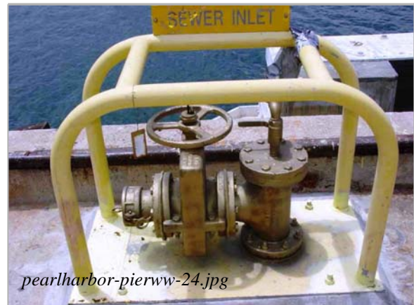
Photo: Pierside - CHT Ships Sanitary Sewer Taken By: Julie Murioka, Navy Region Date: 04/12/06
