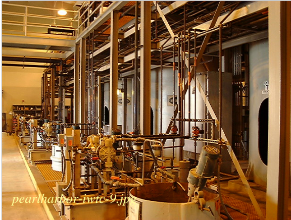
Photo: IWTC - Treatment Reactor Tanks Taken By: Greg V. Arthur Date: 04/10/06
