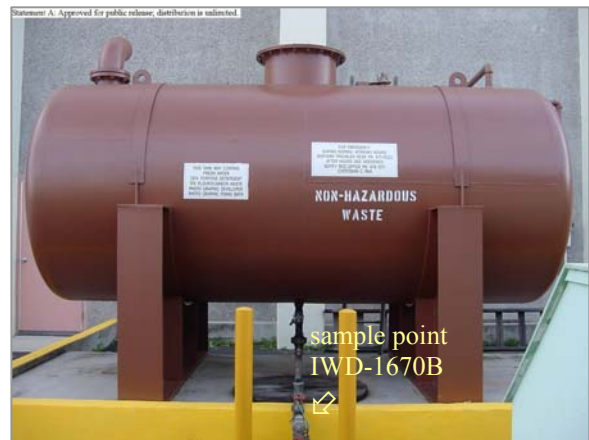
Photo: Bldg 1670 - Tank 1 Discharge to Sewer Taken By: Christie Chun, PHNSY Date: 04/12/06
