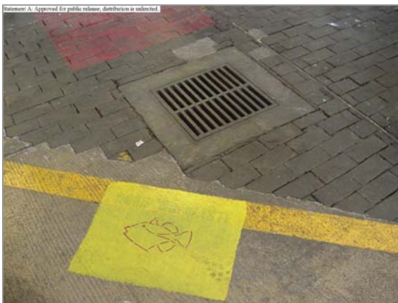
Photo: Bldg 214 - Internal Storm Water Drain Taken By: Christie Chun, PHNSY Date: 04/11/06
