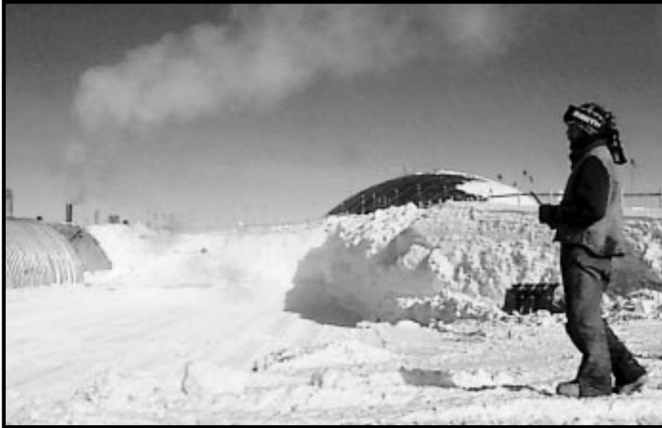
Carlton Walker, ASA Construction Supervisor, watches as D-7 bulldozers move thousands of pounds of snow to make room for a new 200-foot long, 64-foot wide, and 34-foot high garage arch at South Pole Station.
