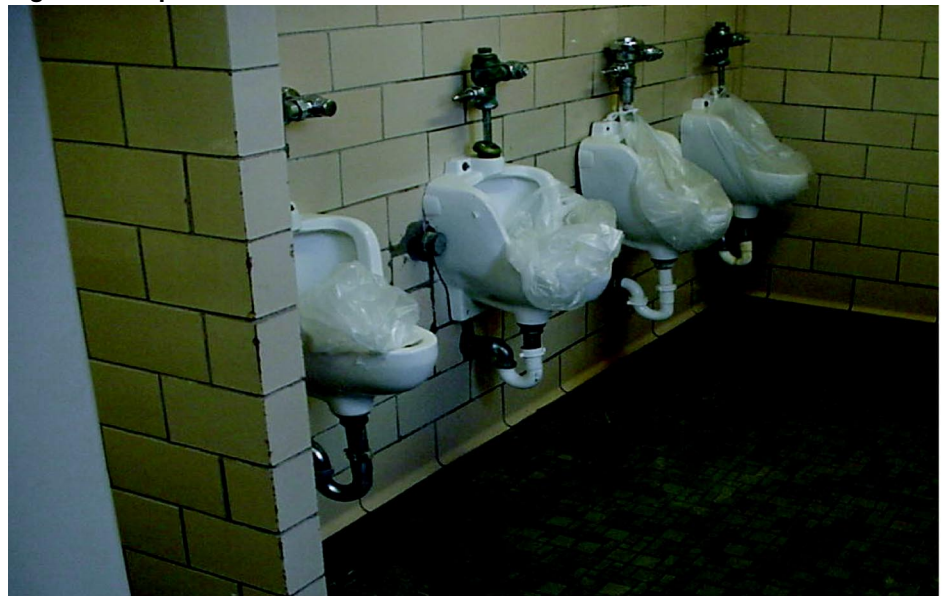
Figure 4: Inoperable Bath Fixtures at Parris Island Recruit Barracks
