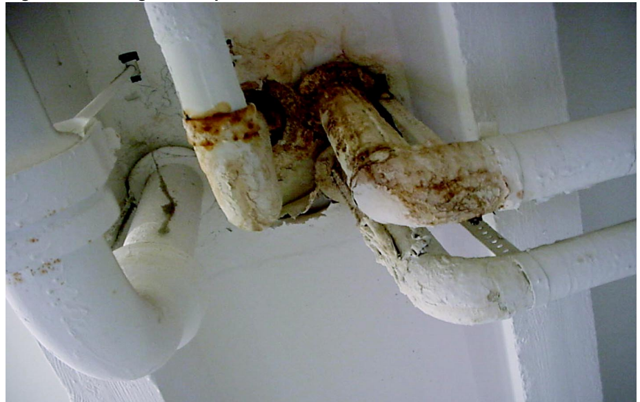
Figure 3: Leaking Drain Pipe at Ft. Knox Recruit Barracks
