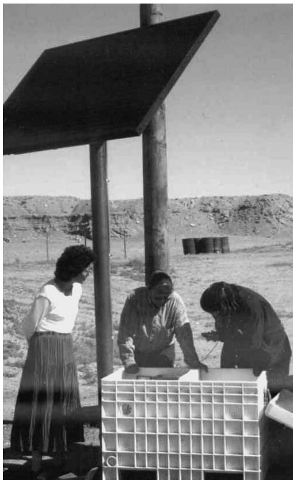
SANDRA BEGAY-CAMPBELL, left, and two Navajo electrical technicians, Vircyntia Charley, center, and Melissa Parrish, check the batteries on a Navajo Tribal Utility Authority photovoltaic system in the Kayenta District, Arizona.
