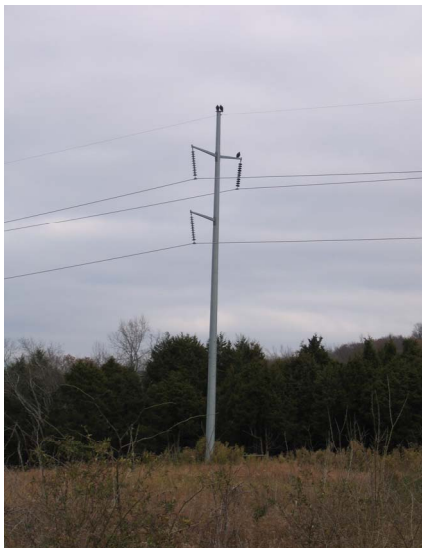
Figure 3. Single Steel Pole 161-kV Transmission Structure
