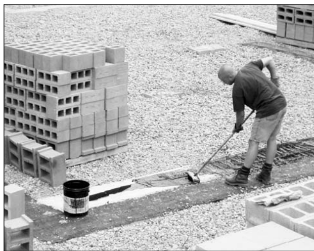
A contractor applies a polymer-enhanced asphalt membrane on top of the footer to act as a capillary break.
