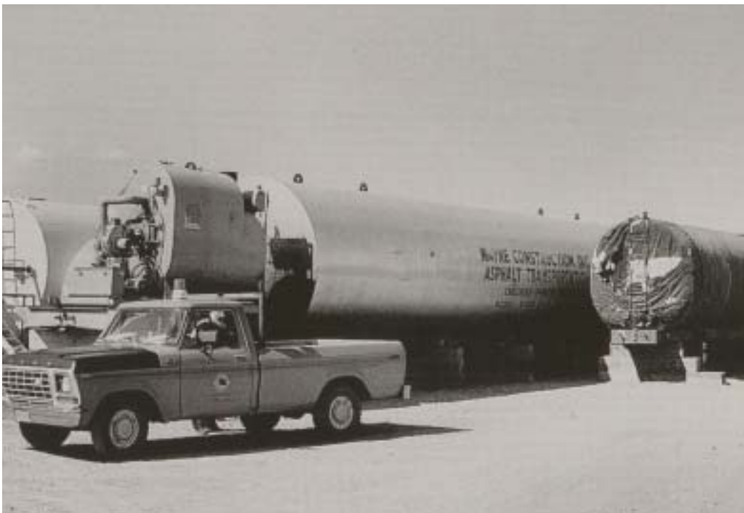
Figure 4-5 Asphalt Cement Storage Tanks
