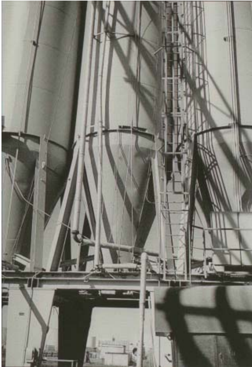
Figure 4-7 Hot Asphalt Storage Silos (The remaining items of Section 4.4 apply only to batch plants)
