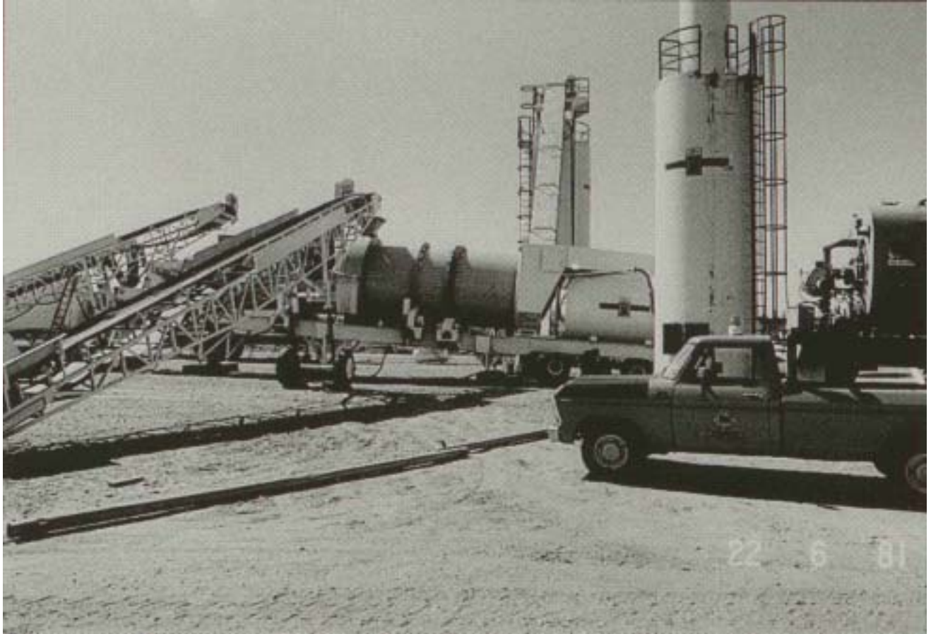
Figure 7-2 Belt to feed RAP into dryer drum
