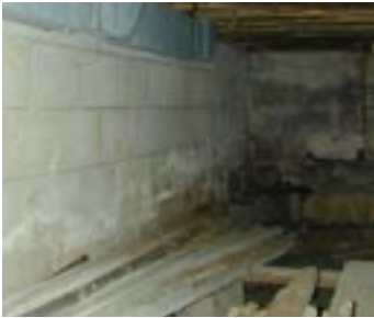
VISIBLE MOISTURE ON THE REAR CONCRETE BLOCK IN THIS CRAWLSPACE CAN CONTRIBUTE TO MOLD GROWTH IF NOT ABLE TO DRY. WHITE STAINS ON THE SIDE WALL ARE INDICATIVE OF PREVIOUS MOISTURE PROBLEMS.
