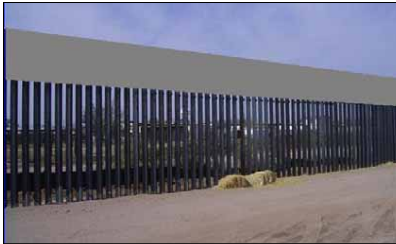
Figure 1-2. Personnel-Vehicle Fence Type-1 (PV-1)
