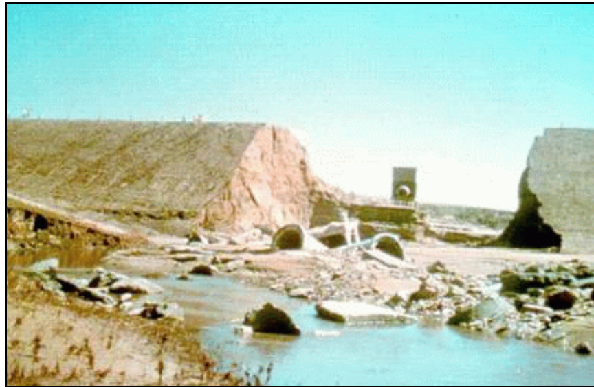
Figure 6. —Embankment dam failure caused by internal erosion of earthfill near the conduit. The initial failure was tunnel shaped, but the collapse of the roof of the tunnel resulted in the observed shape of breach. Hydraulic fracture in highly dispersive clay embankment soils caused the failure. The embankment dam design included antiseep collars, but no filter diaphragm.
