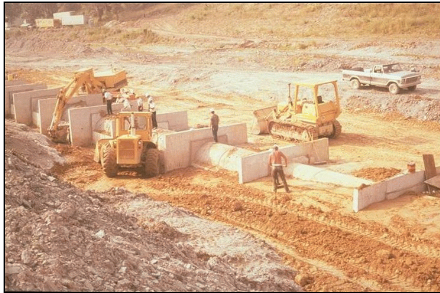
Figure 14. —Antiseep collars impeded the compaction of soils around the conduit. Hand tampers were used next to the antiseep collars.
