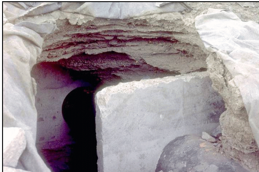
Figure 18. —Antiseep collars were not adequate to prevent the internal erosion failure of this embankment dam. The internal erosion that occurred on first filling of the reservoir occurred in dispersive clay soils that are not susceptible to backward erosion piping.
