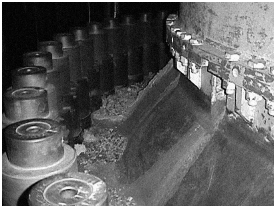
Figure 5: Rust and Boric Acid on Davis-Besse's Vessel Head as Shown to Resident Inspector during the 2000 Refueling Outage
